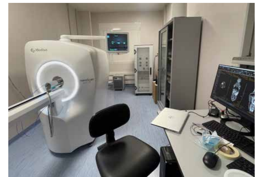
nanoScan® MRI 7T reference installation with every system component (magnet, workstation, electronic cabinet, He-compressor, chiller) located in the same imaging room.
